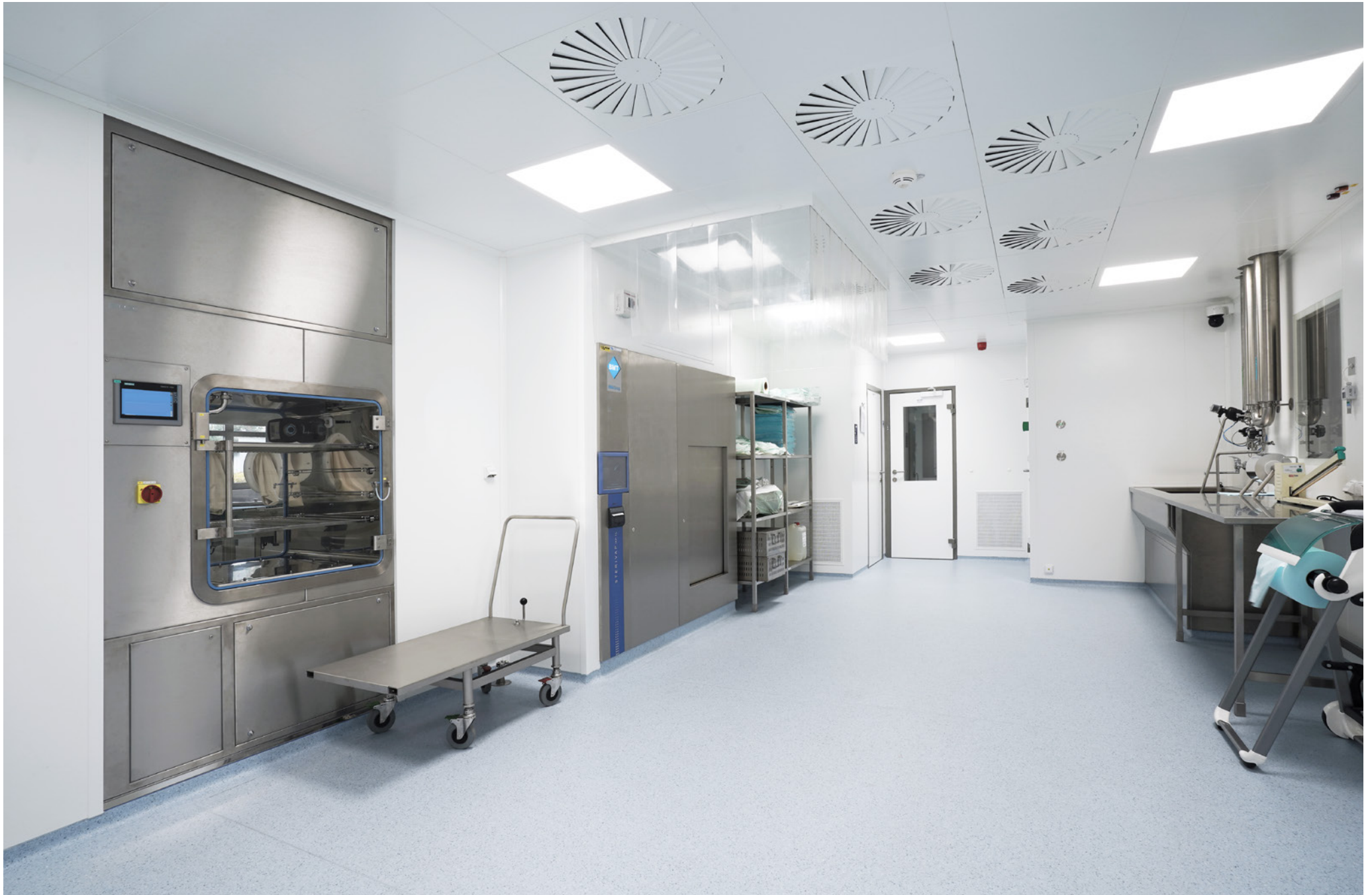
VHP Decontamination Lock | Bioveta | Czech Republic
