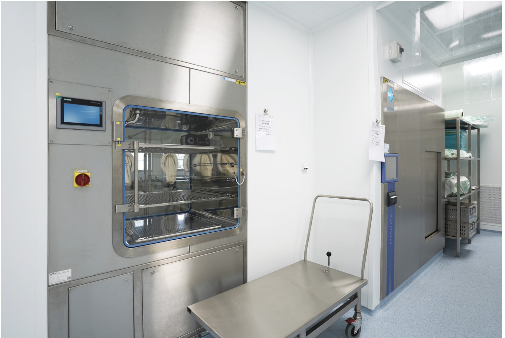
VHP Decontamination Lock | Bioveta | Czech Republic
