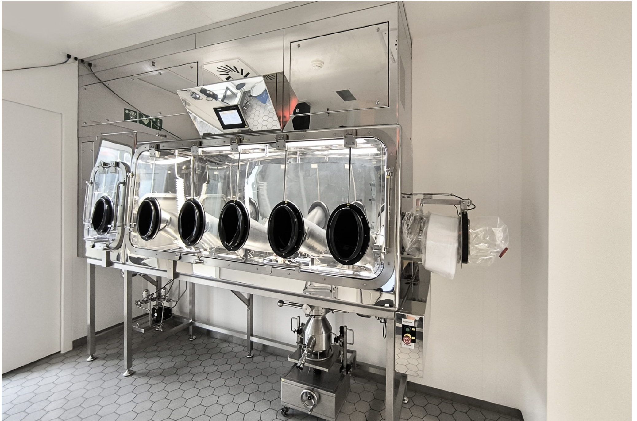
Dispensing Isolator | Merck & Cie KmG | Switzerland
